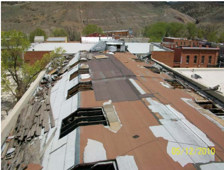
Penetrations in the roof to install shoring remain, allowing moisture to enter the building
