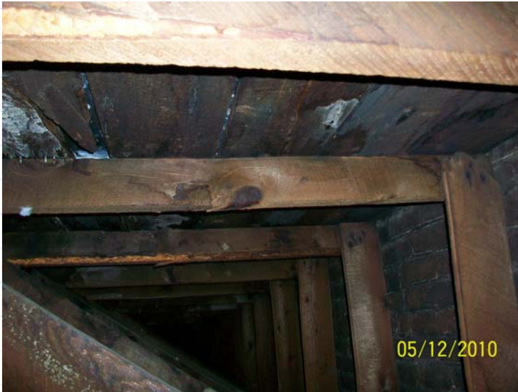
Roof/Wall Connection – no rim joist/bolting/attachment noted to brick wall at right
