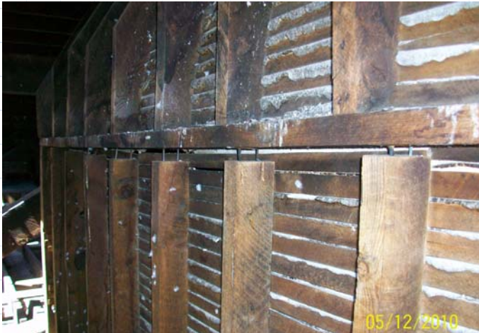
Skylight wall –note gap where studs are pulling away from plate due to cracked beam
