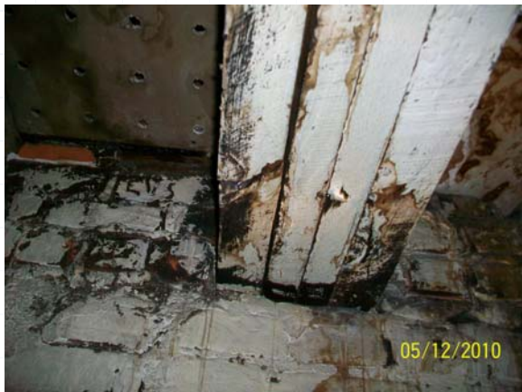
Truss #6, South Bearing – note crack in bottom of left member
