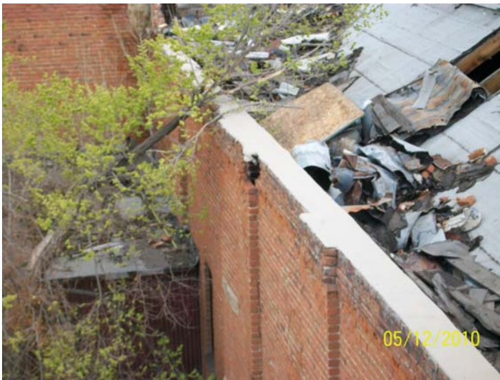
Hole in top of wall allows water to enter cavity between wythes of brick
