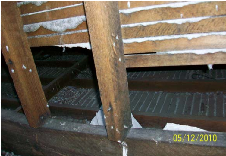
Beam supporting skylight wall – note crack in beam at lower left allowing excessive deflection
