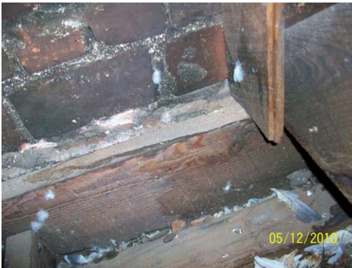
Ceiling rim joist – no attachment observed
