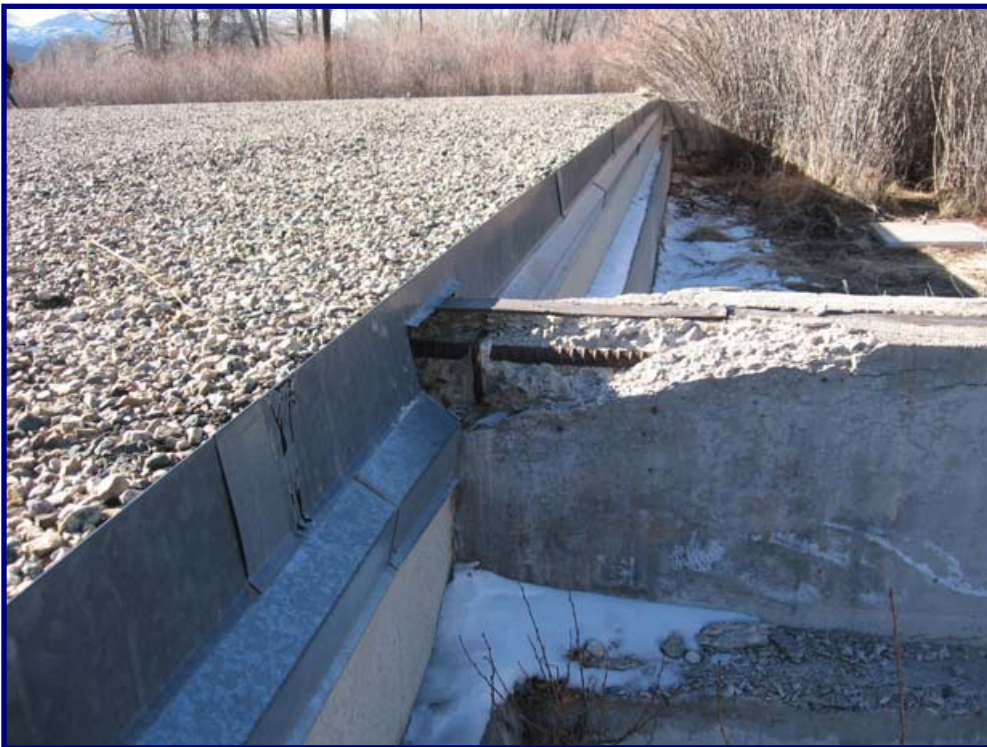
Photo 4 - Inverted Tee Beam – Spalled concrete/corroded reinforcement
