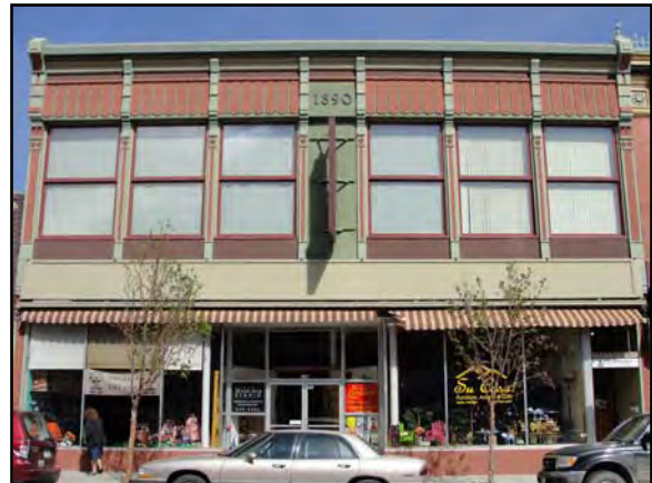
134 F Street, Disman-Alger Block – Original second story windows and cornice had been previously removed. Replacements were created in the scale of the original, but not identical materials or design.
