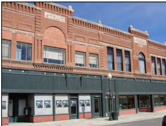
230 F St, McKenna Building – The left side of the building has undergone an inappropriate window replacement.
