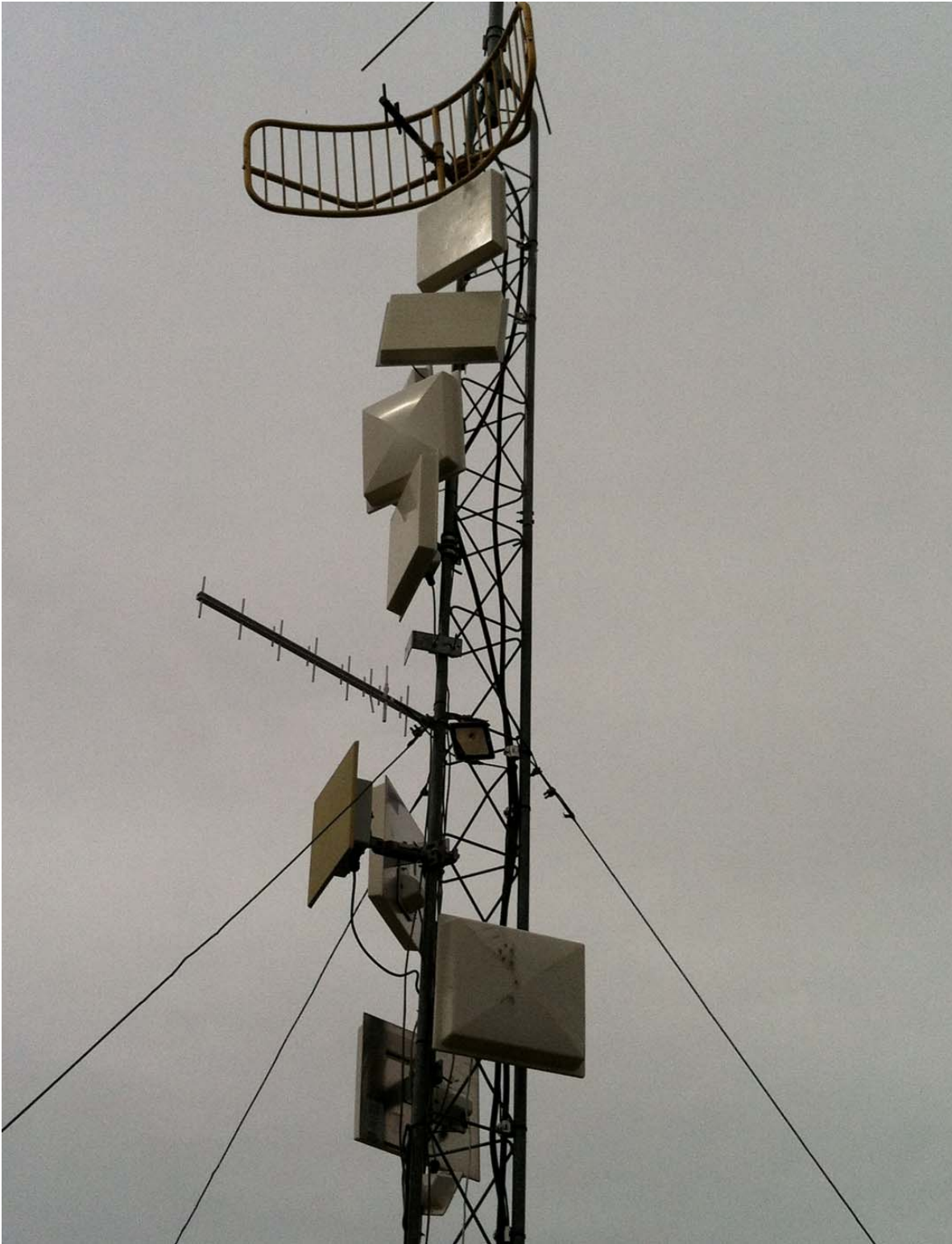
Existing (KHEN) 30 ft. tower on Tenderfoot Mountain.
